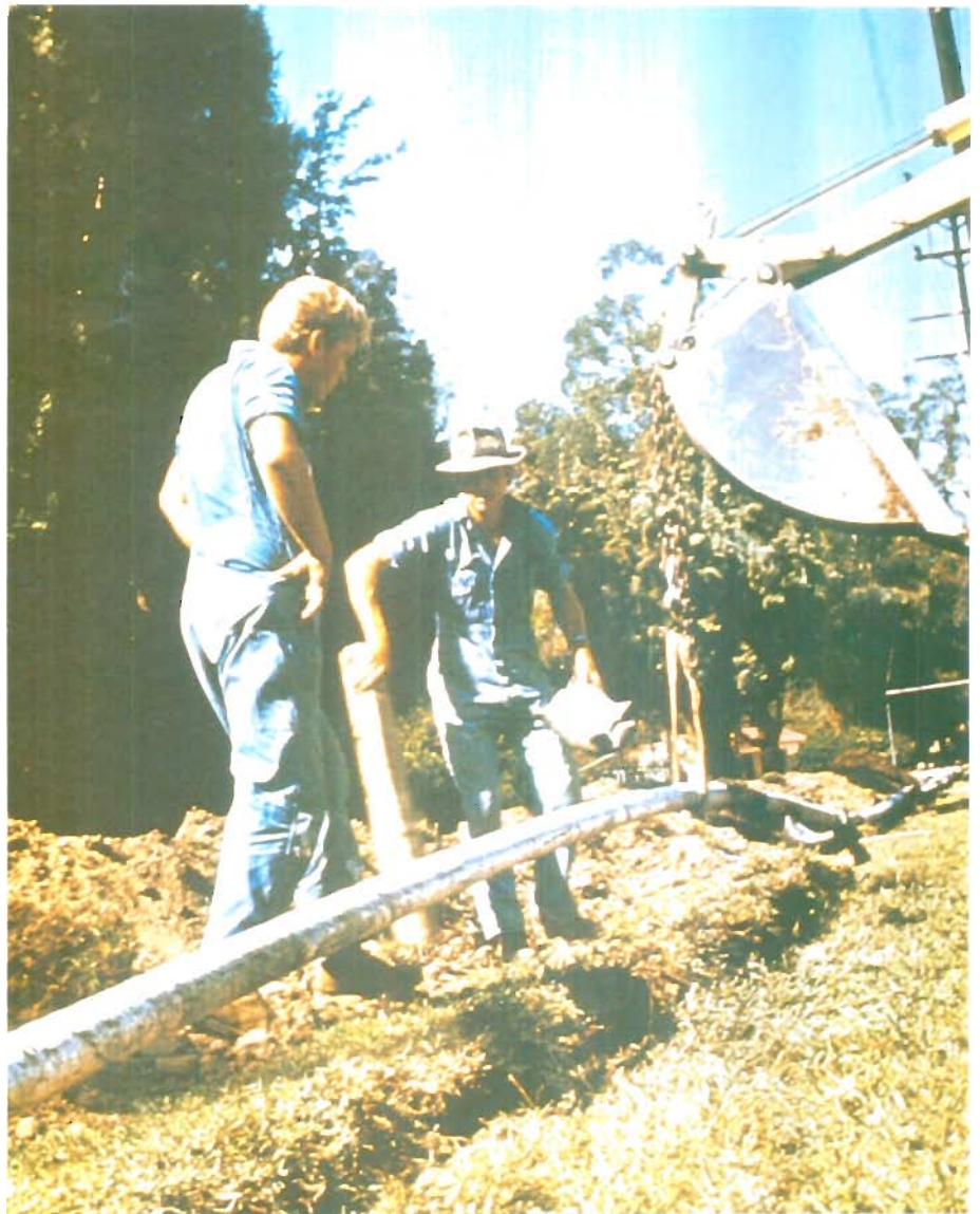
Gas company workers labor to install a delivery line in the complex network needed to transport the fuel to customers. Workers depend upon accurate tract maps to make their efforts safe and efficient.
